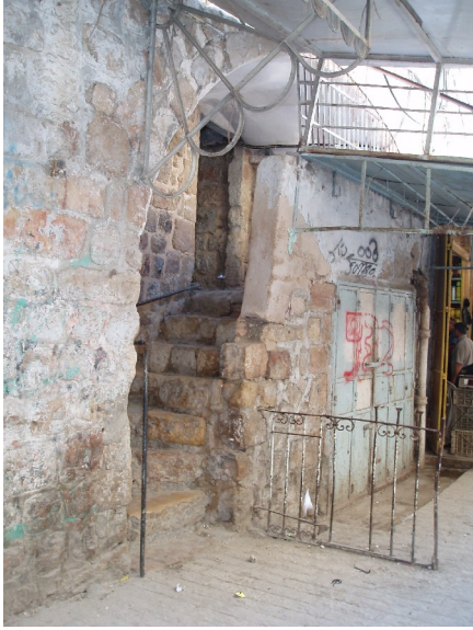
(Picture 5.1) Broken access: an entrance of an old city house (source: the researcher)
